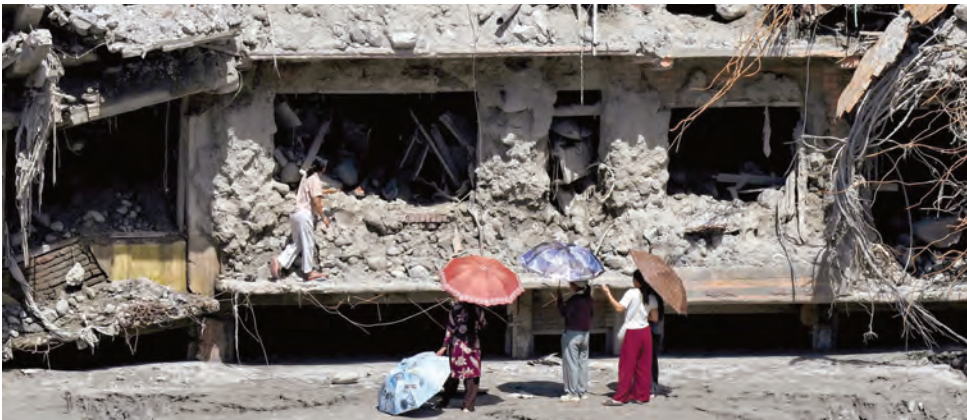
People look at a house, damaged during the August 26 flash flood, at Trishuli in Nepal’s Nuwakot district. — AFP file photo
