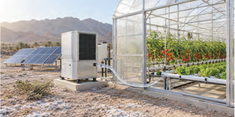
Depending on weather conditions and machine capacity, the systems were able to produce up to 40 or 100 litres of water per day.
