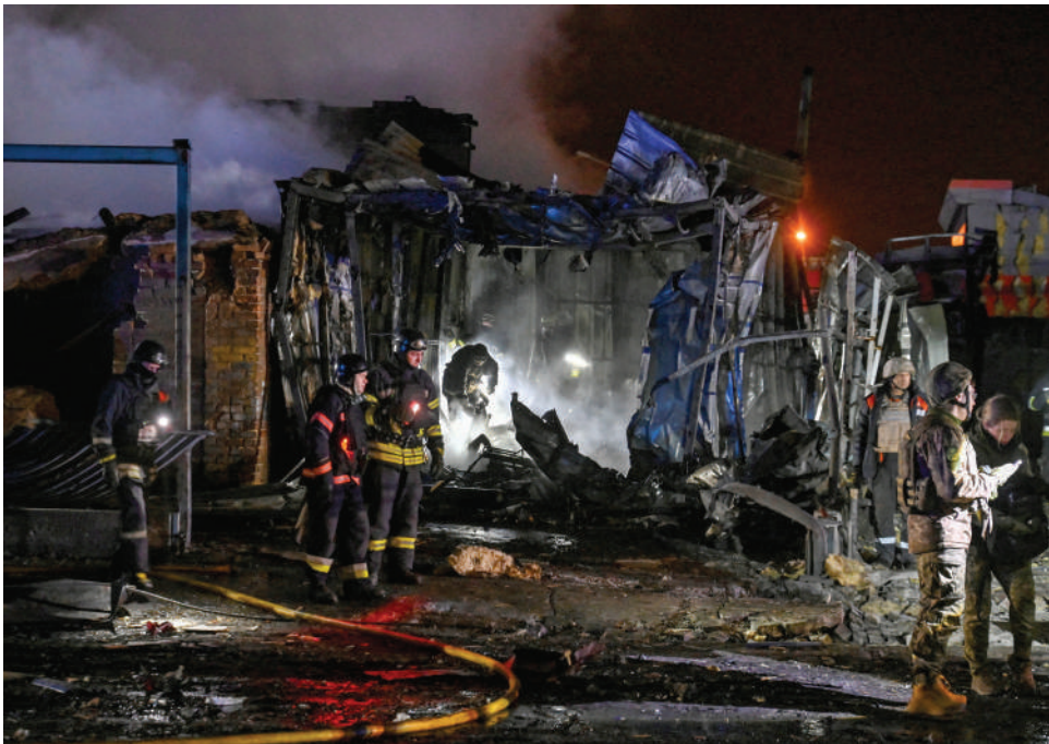
Firefighters work at the site of a car maintenance workshop heavily damaged by a Russian air strike, in Zaporizhzhia. — Reuters
