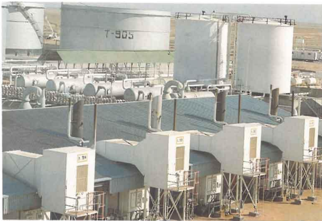
Gas turbines at Yibal – Oman is self-sufficient in natural gas (Photo: P.D.O.)
