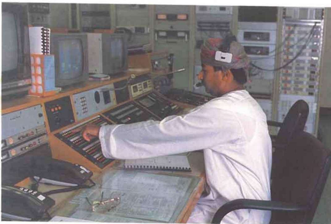
Oman Radio's master control room
