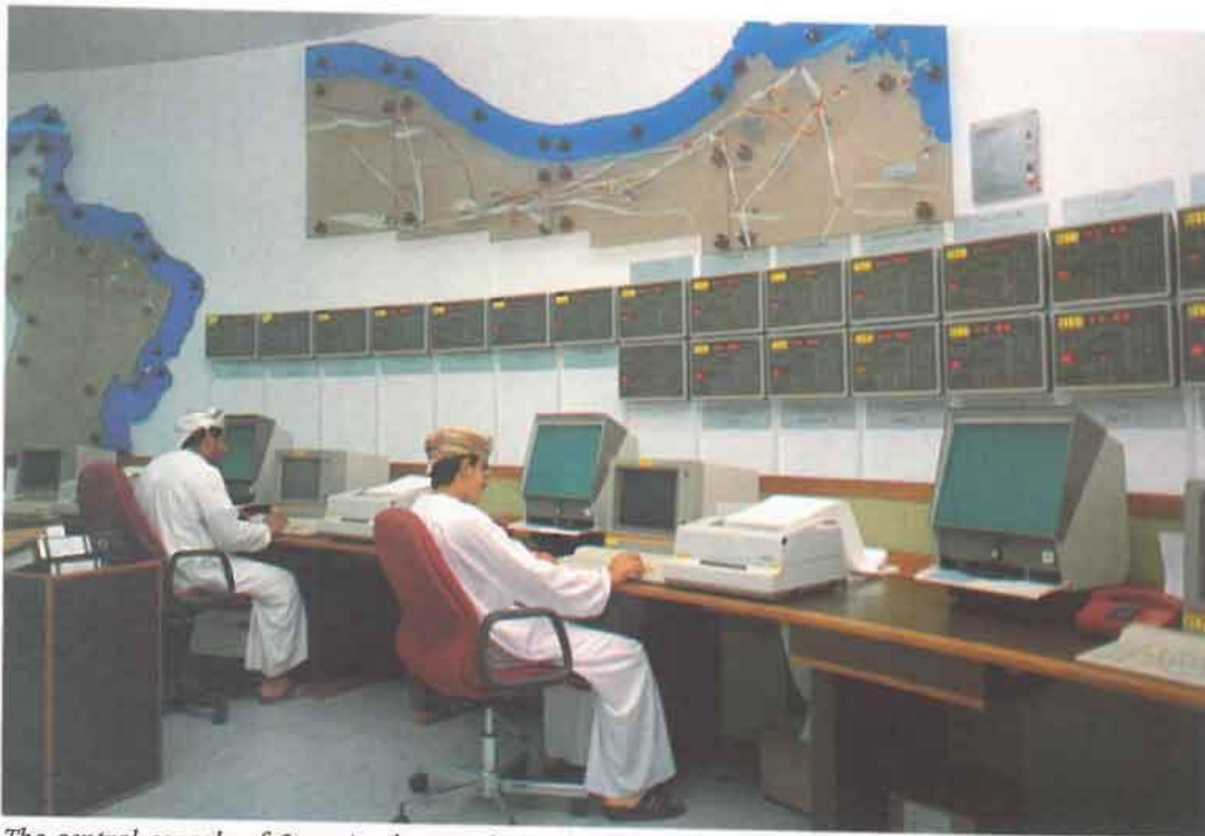
The central console of Oman's ultra-modern telephone system
