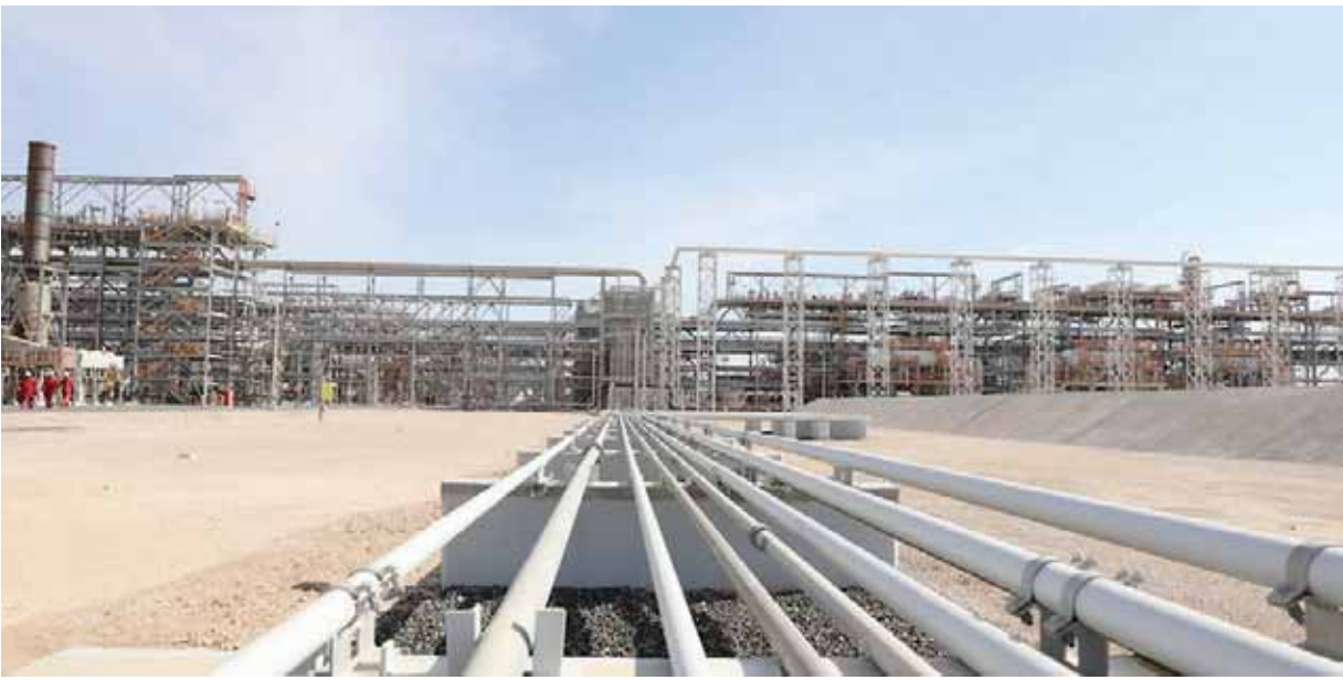
Gas production facility pictured in Oman.
