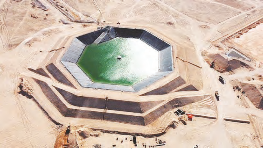
The Rima Wetlands use natural wetlands integrated with physical, biological treatment processes to handle 66,000 cubic metres of oily produced water daily.
