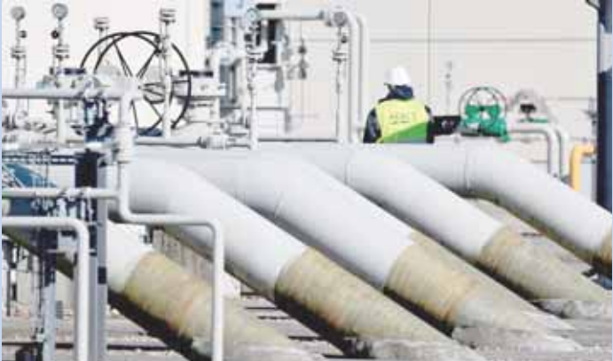
A man is seen inside landfill facilities of the Nord Stream 1 gas pipeline in Lubmin, Germany. – Reuters
