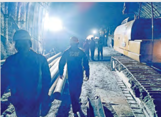
Rescue workers are seen at the site after a tunnel collapsed in the Uttarkashi district of India's Uttarakhand state, on Monday (AFP)
