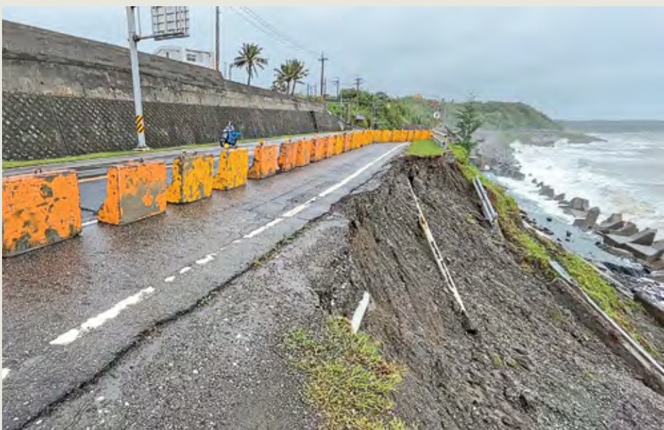
A damaged section of highway is seen in the aftermath of Typhoon Haikui in Taitung County on Monday (AFP)
