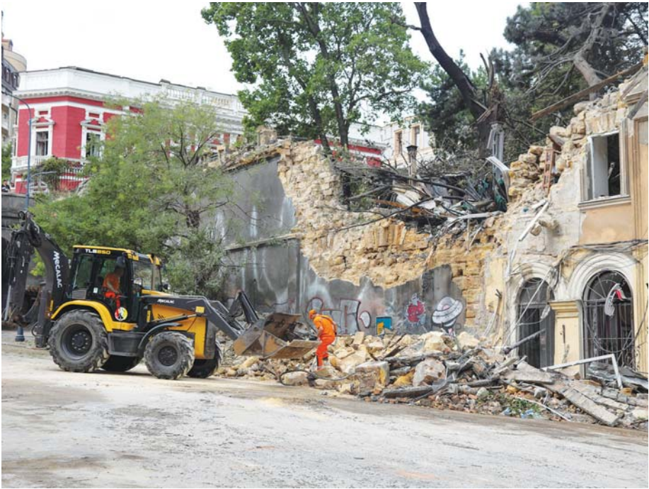
Municipal workers remove debris at a site of a building damaged during Russian missile strikes, amid Russia's attack on Ukraine, in Odesa. — Reuters
