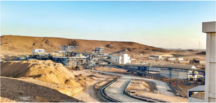
New copper concentrator plant currently under commissioning at the Washihi site.
