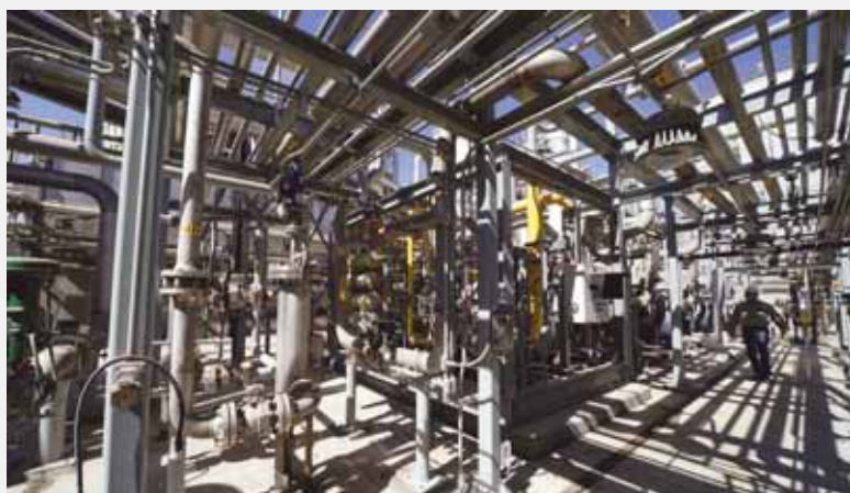
Calgren’s renewable fuels facility that cleans dairy methane into natural gas is shown in Pixley, California. — Reuters
