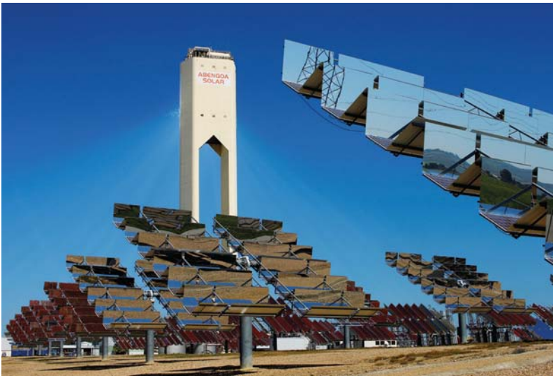
A tower and solar panels belonging to the Abengoa are seen at the Solucar solar park in Sanlucar la Mayor, near the Andalusian capital of Seville, Spain. – Reuters
