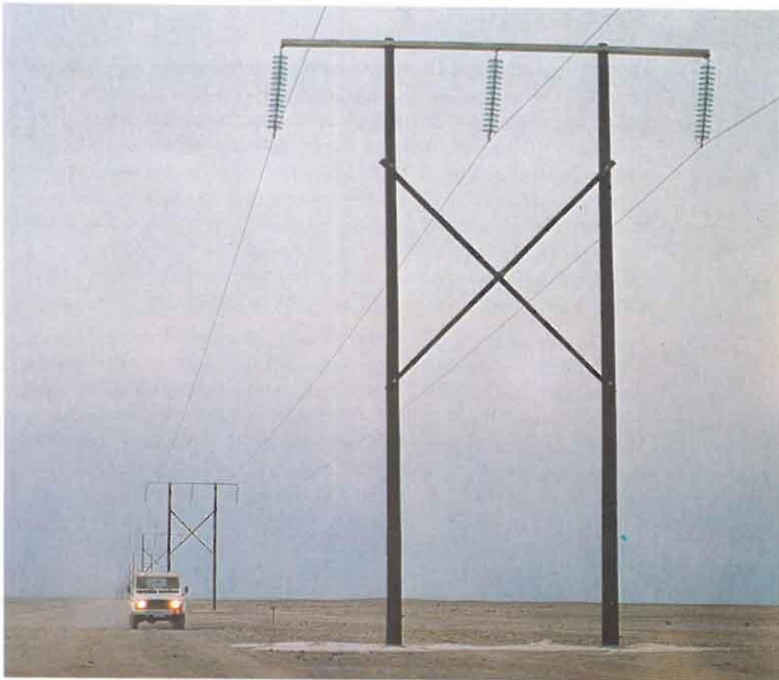
Part of the Sultanate's extensive national power grid (Photograph: PDO)
