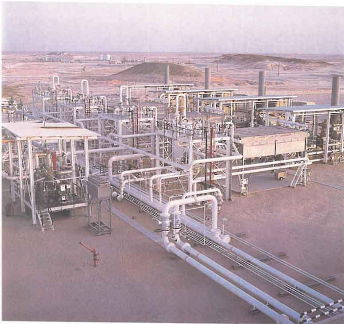
PDO's gas plant at Yibal (Photograph: PDO)
