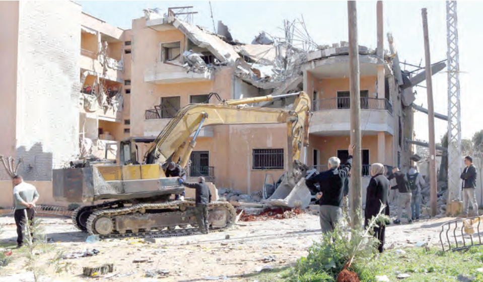
An excavator clears rubble before a heavily-damaged building in the centre of Lebanon’s eastern Bekaa Valley region. — AFP
