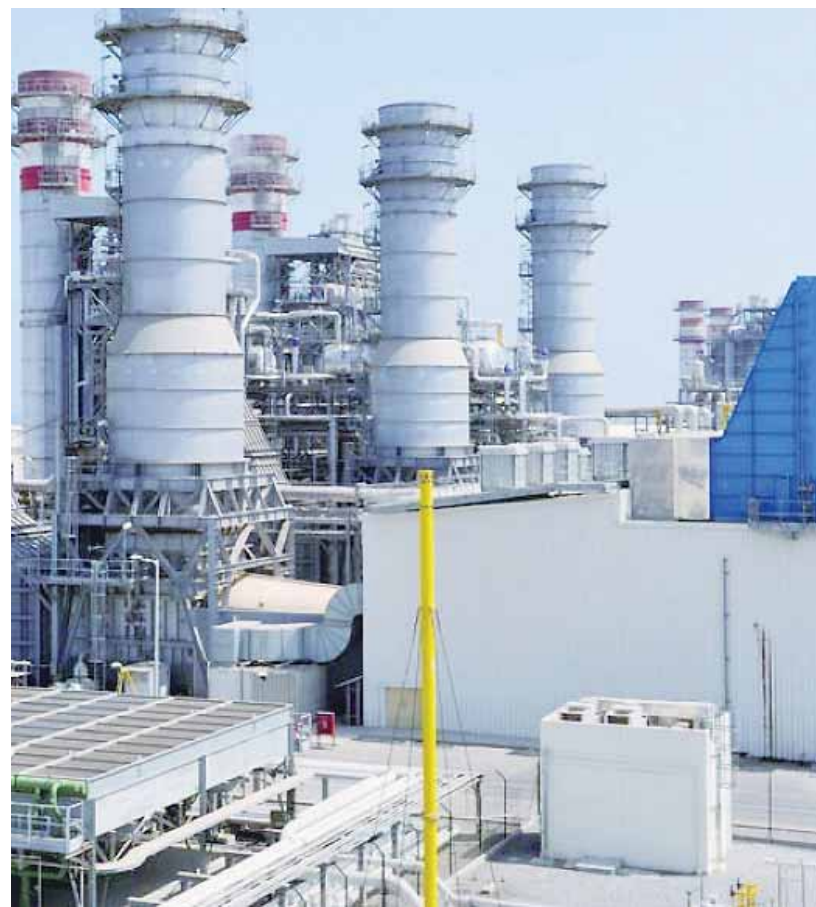
SMN Power is a significant player in Oman's power and water sector.
