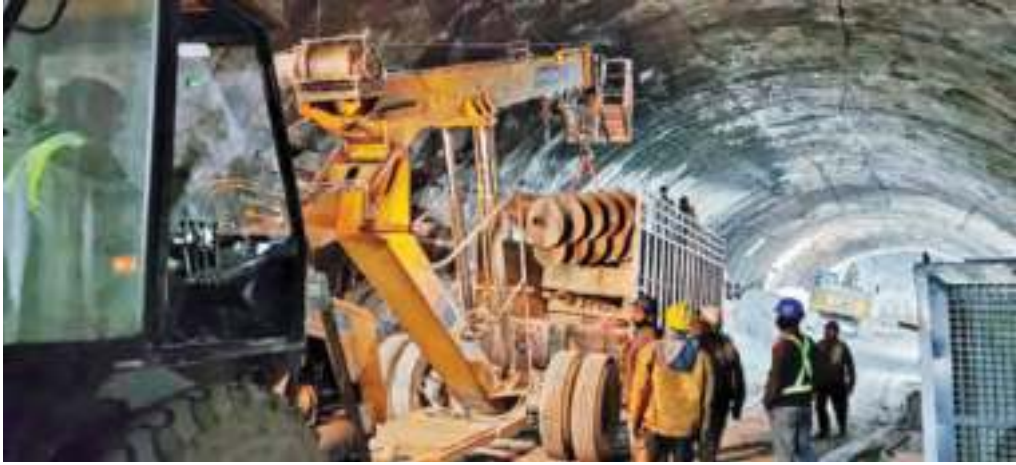
SDRF personnel are seen inside tunnel which collapsed, in Uttarkashi, India on Tuesday (ANI)
