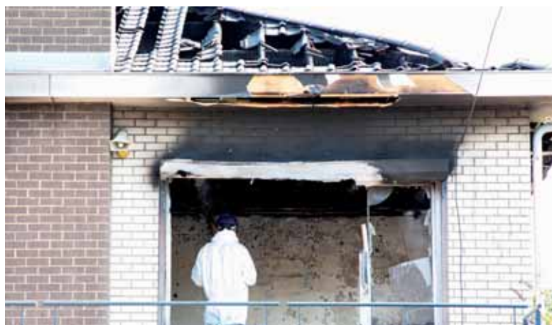
A forensic inspector inspects a house where a fire killed five people in Ville-sur-Haine, Belgium. — AFP
