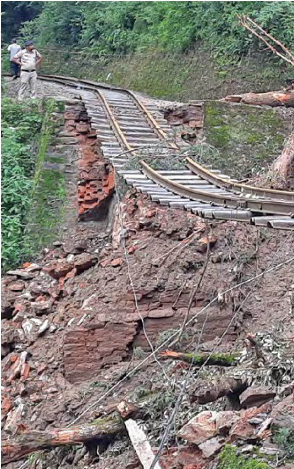
A view of damaged Shimla-Kalka railway track, an UNESCO world heritage, after 50 metres of a bridge was swept away due to landslides caused by incessant rains near Summer Hill on the outskirts of Shimla, India, on Wednesday (AFP)
