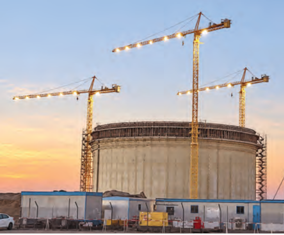
Marsa LNG's 165,000-cubic-metre LNG storage tank is entering the final stages of completion.
