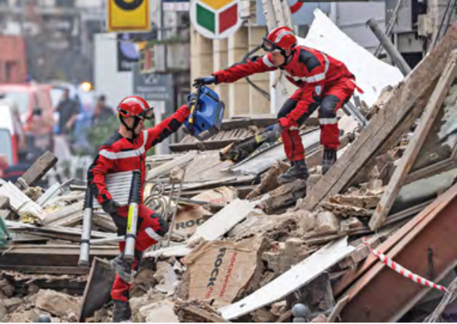
Firefighters inspect a collapsed building as they search for victims in the city of Lille, northern France, on Saturday (AFP)
