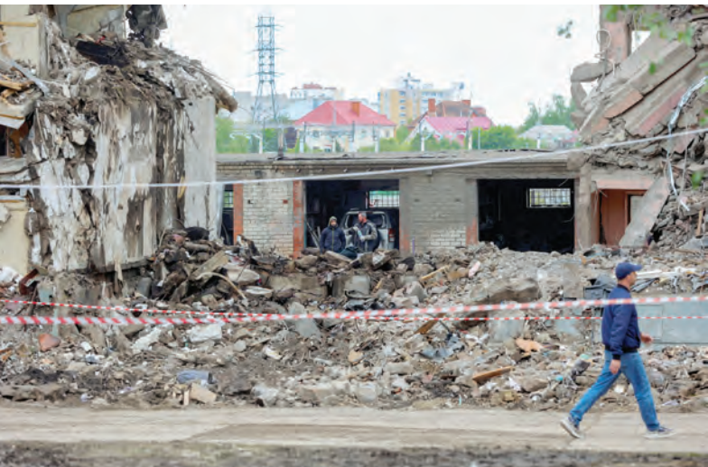
Workers remove debris of a damaged multi-storey apartment block, in the city of Belgorod. — Reuters
