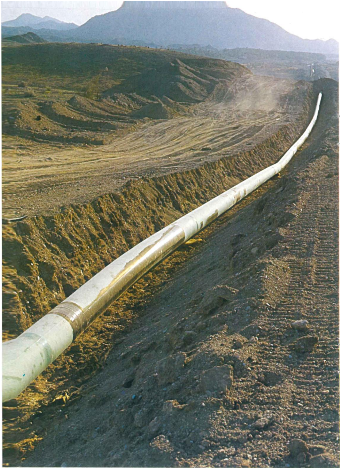
Pipeline carrying natural gas which is providing Oman's industries with cheaper energy.
