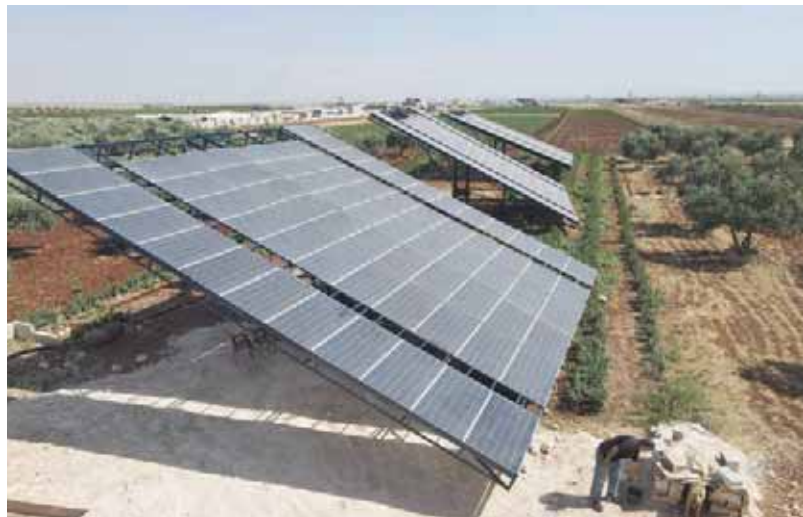
Solar panels are installed in agricultural fields, in the village of Killi, near Bab al Hawa by the border with Turkey, in Syria’s northwestern Idlib province. – AFP
