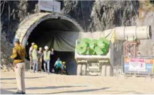
A supply truck loaded with augers prepares to enter a tunnel where 40 road workers are trapped after a portion collapsed in Uttarkashi in the northern state of Uttarakhand, India. – Reuters
