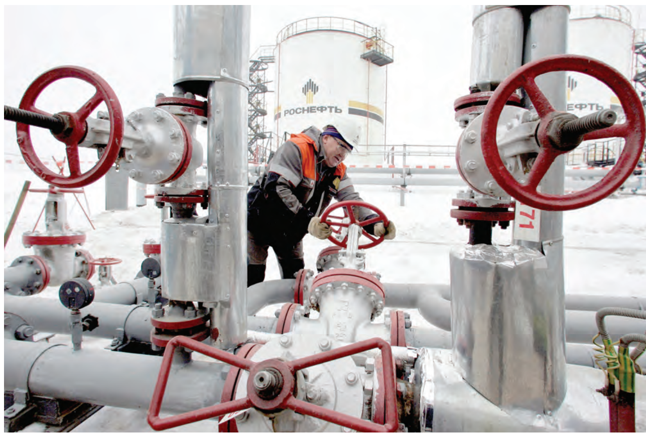
A worker turns a valve at UdmurtNef't's Gremikhinskoye oil field east of Izhevsk near the Ural Mountains, Russia. – Reuters
