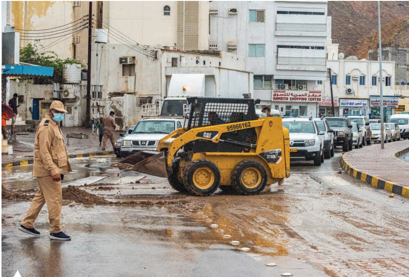
Hamriya Muscat Municipality swiftly deployed teams to clear debris from roads
