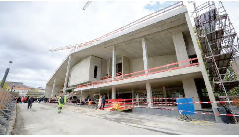
The opening of a new museum in the German capital, the Berlin Modern, has been delayed again to 2030 after water damage and microbial infestation were discovered in parts of the building — DPA
