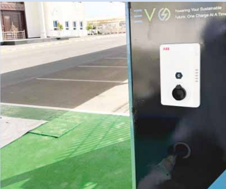
An EV-friendly car parking slot with charging infrastructure.
