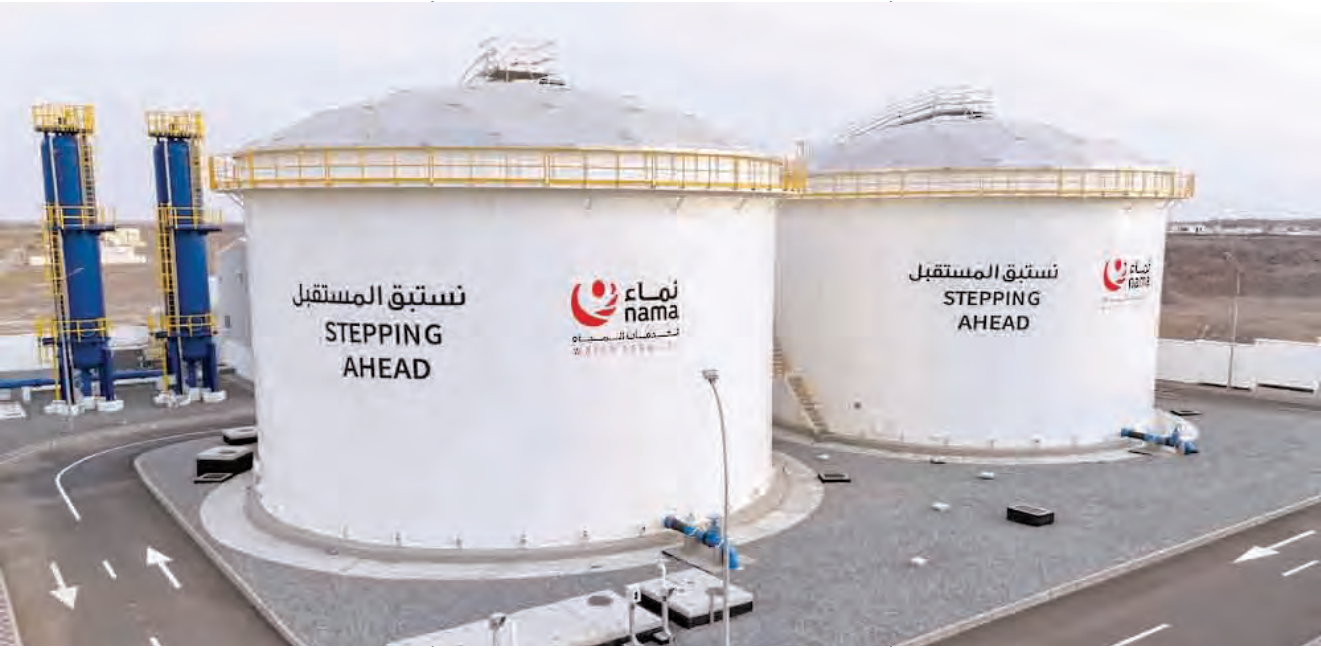
The 1.41 million m³/day capacity is supported by 61 desalination plants, alongside 115 pumping stations, 922 reservoirs and tanks, 475 tanker filling stations and 865 wells.
