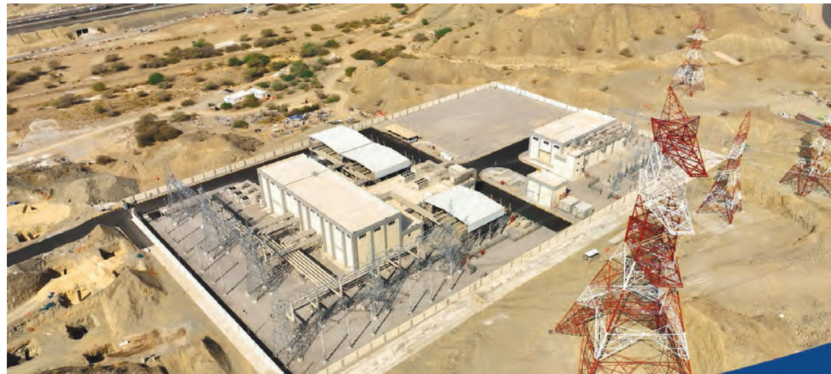
OETC is making substantial investments in upgrading Oman's power transmission system.
