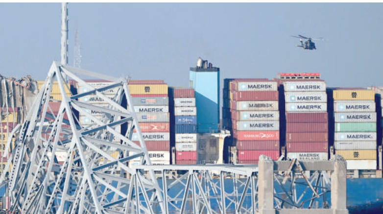
The remains of the collapsed Francis Scott Key Bridge lie in the Patapsco River after the container ship Dali (L) struck it on March 26. — AFP file photo
