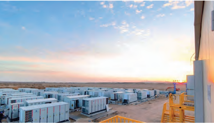
Each BESS project has a storage capacity of 500 MW/2,000 MWh, enabling it to deliver 500 MW of electricity for four hours.
