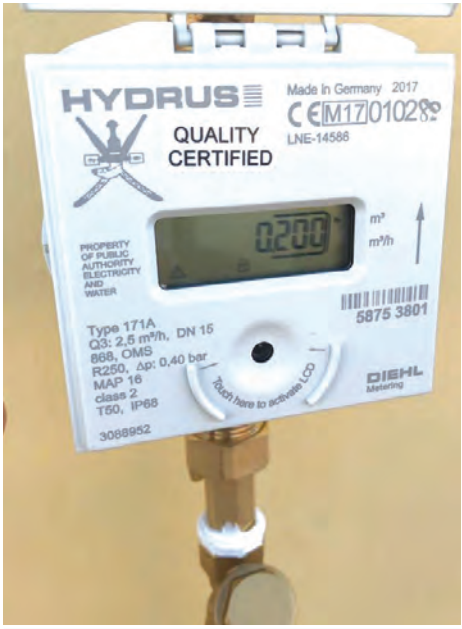
Nama Water Services is implementing a phased plan to complete the smart meter rollout.
