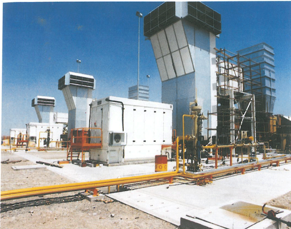
▲ A new power station - many will be powered by gas from Oman's fields in the future.
