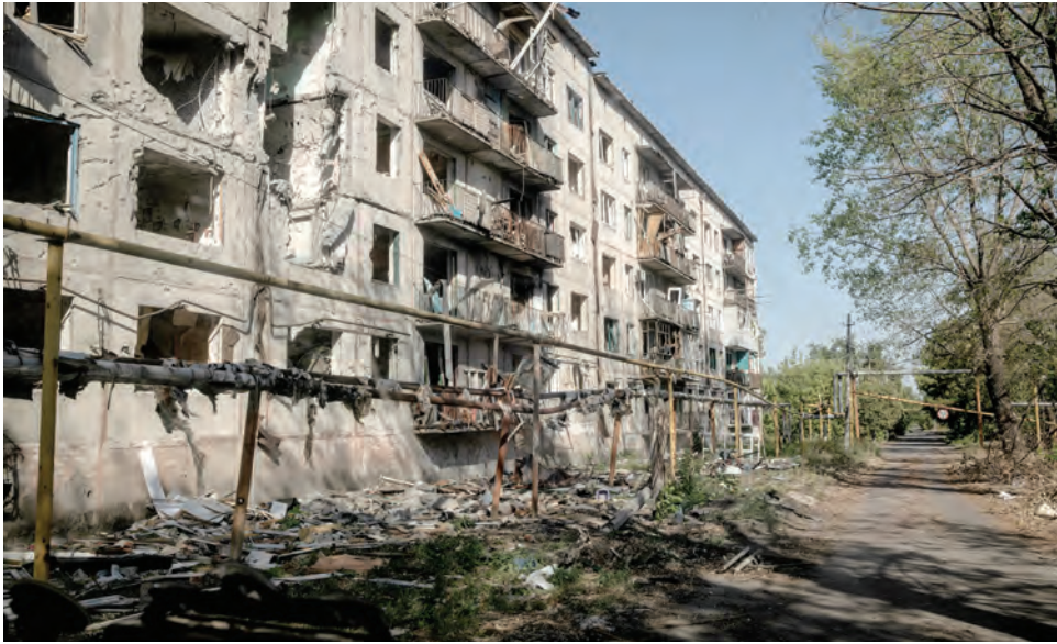
A heavily damaged residential building, caused by Russian strikes, in Myrmohrad, Ukraine.
