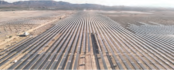
The Al Kamil Solar IPP will add 280 MW of renewable energy capacity to the national grid. Image for illustration only.
