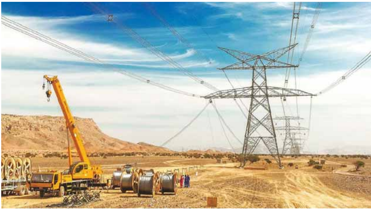
To facilitate the development of new production capacities, Oman has initiated the Rabt project.
