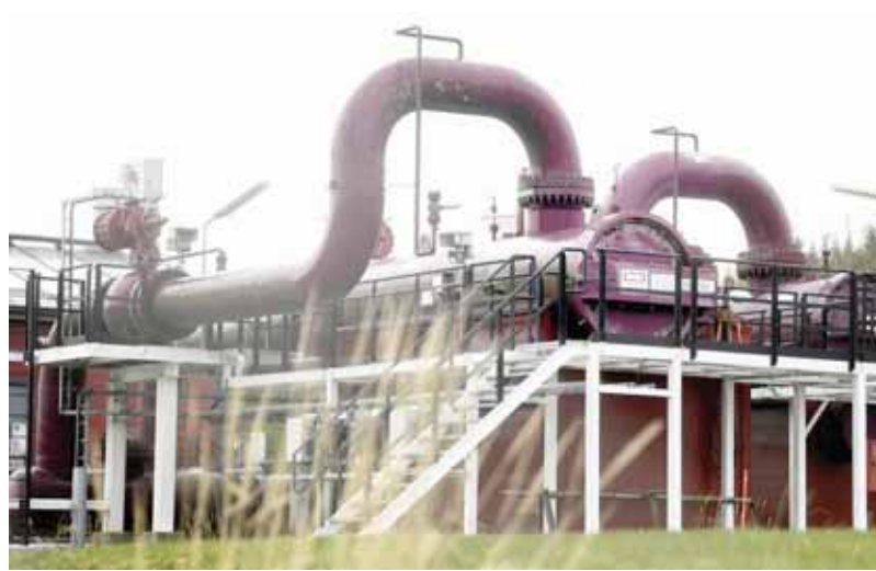
Gas pipes at the Gasum plant are pictured in Raikkola, Imatra, Finland. — AFP
