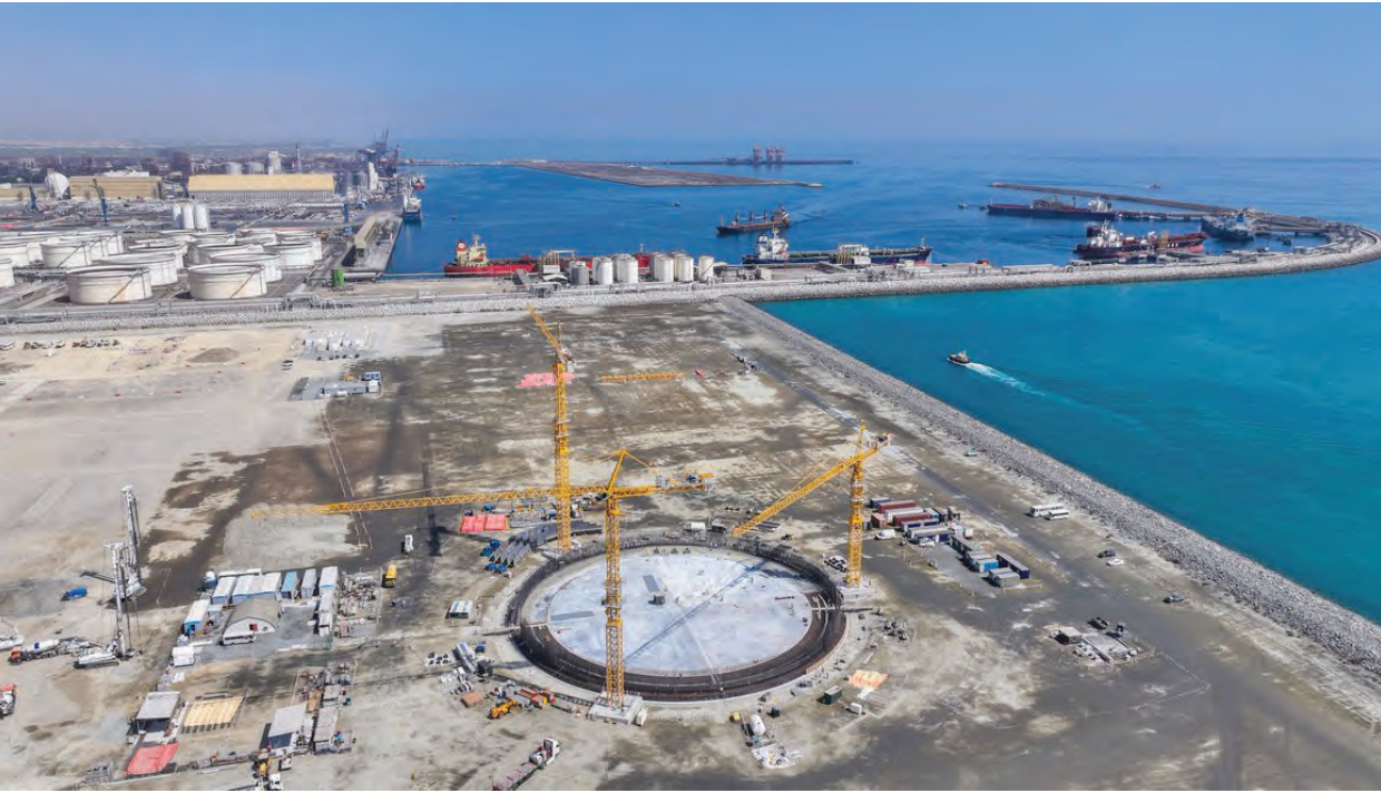
Marsa LNG represents an investment in the future of Sohar Port as a hub for energy and maritime services.
