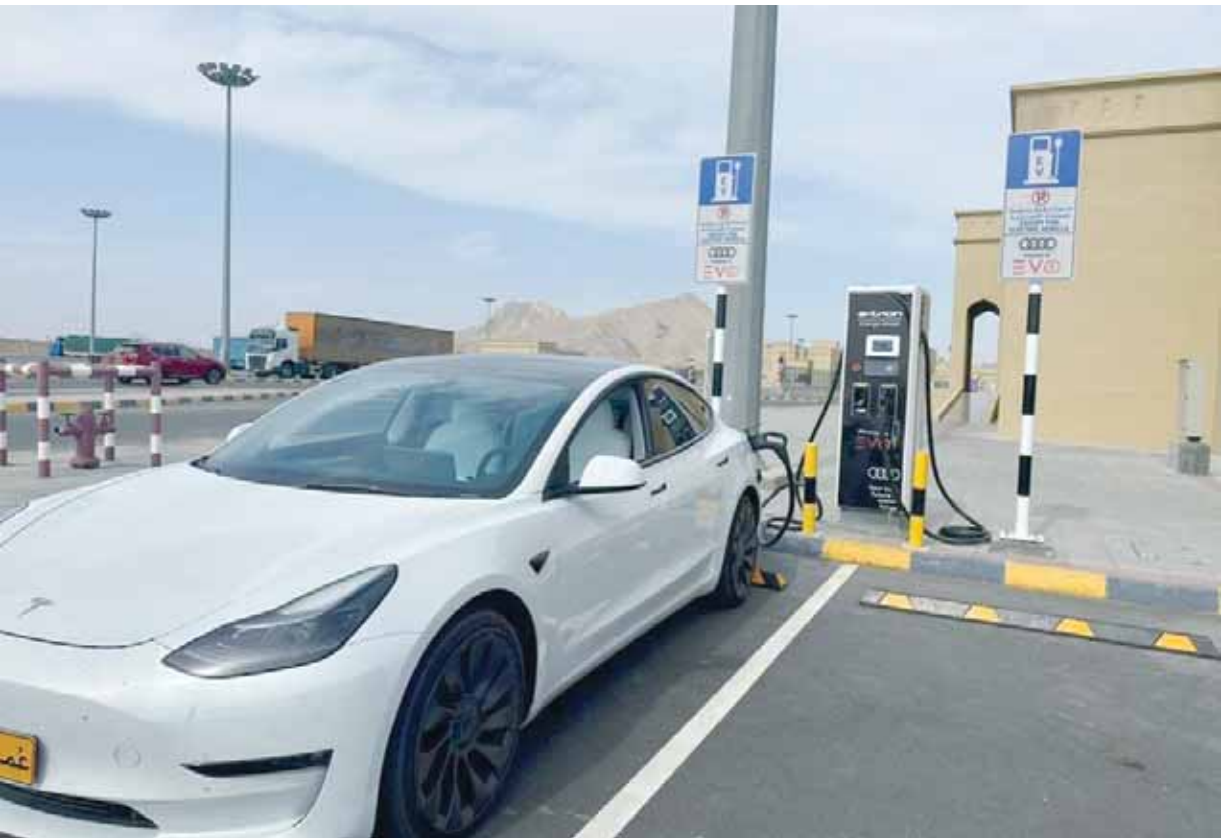
Major ramp-up of EV charging infrastructure on anvil
