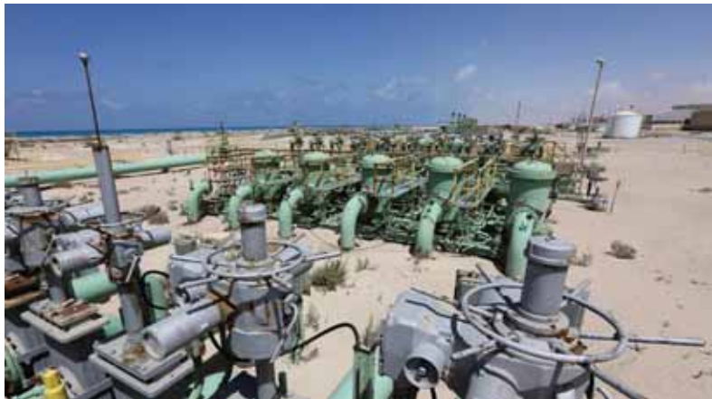
A general view of pipelines at an oil terminal is seen in Zueitina, Libya. — Reuters
