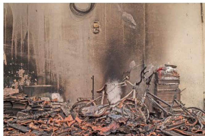
A house stands completely charred following a wildfire engulfing the village of Kastri on Evia (Euboea) Island, on Tuesday (AFP)
