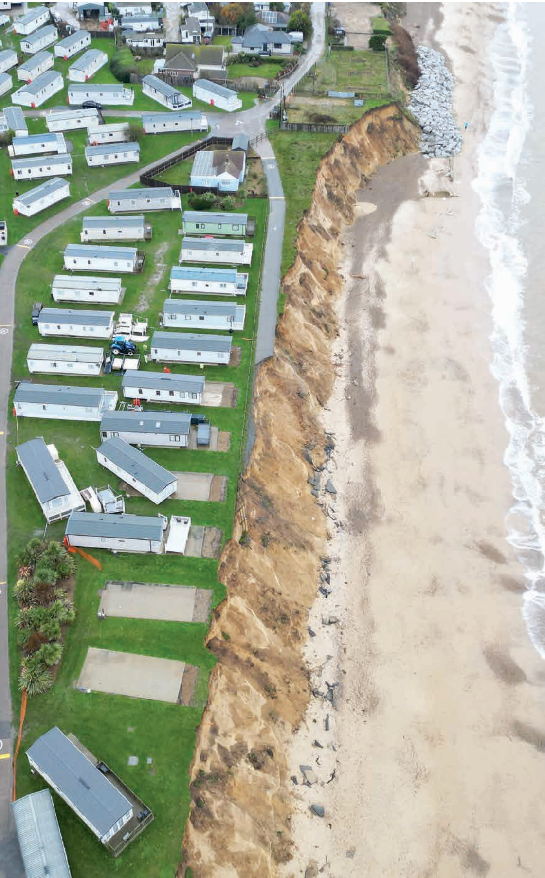
View of the seafront and collapsed road following the erosion caused by high tides and wind at Pakefield Holiday Park in Lowestoft, Britain, on Tuesday. – Reuters
