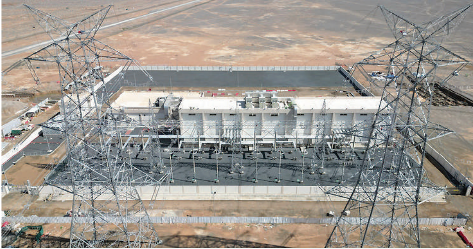
The grid station will evacuate power from a new wind IPP to come up at Jaalan Bani Bu Ali in Al Sharqiyah South Governorate.
