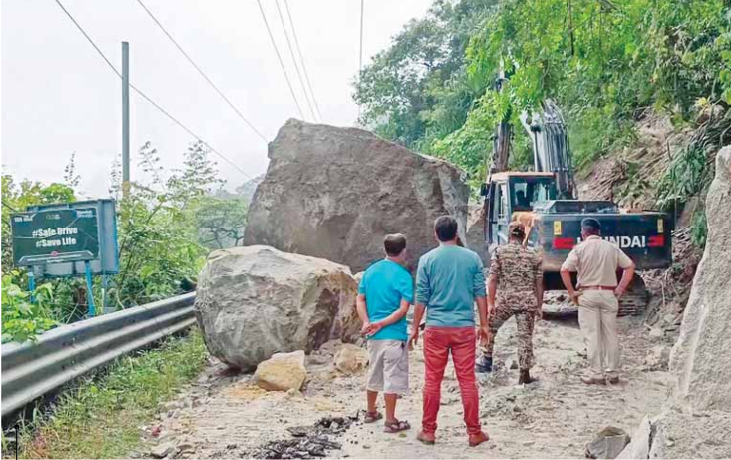
ROAD CLEARANCE WORK IS UNDERWAY AFTER A LANDSLIDE: Road clearance work is underway after a landslide triggered by incessant rainfall at Kalijhora along NH 10, in Kalimpong. — ANI video grab
