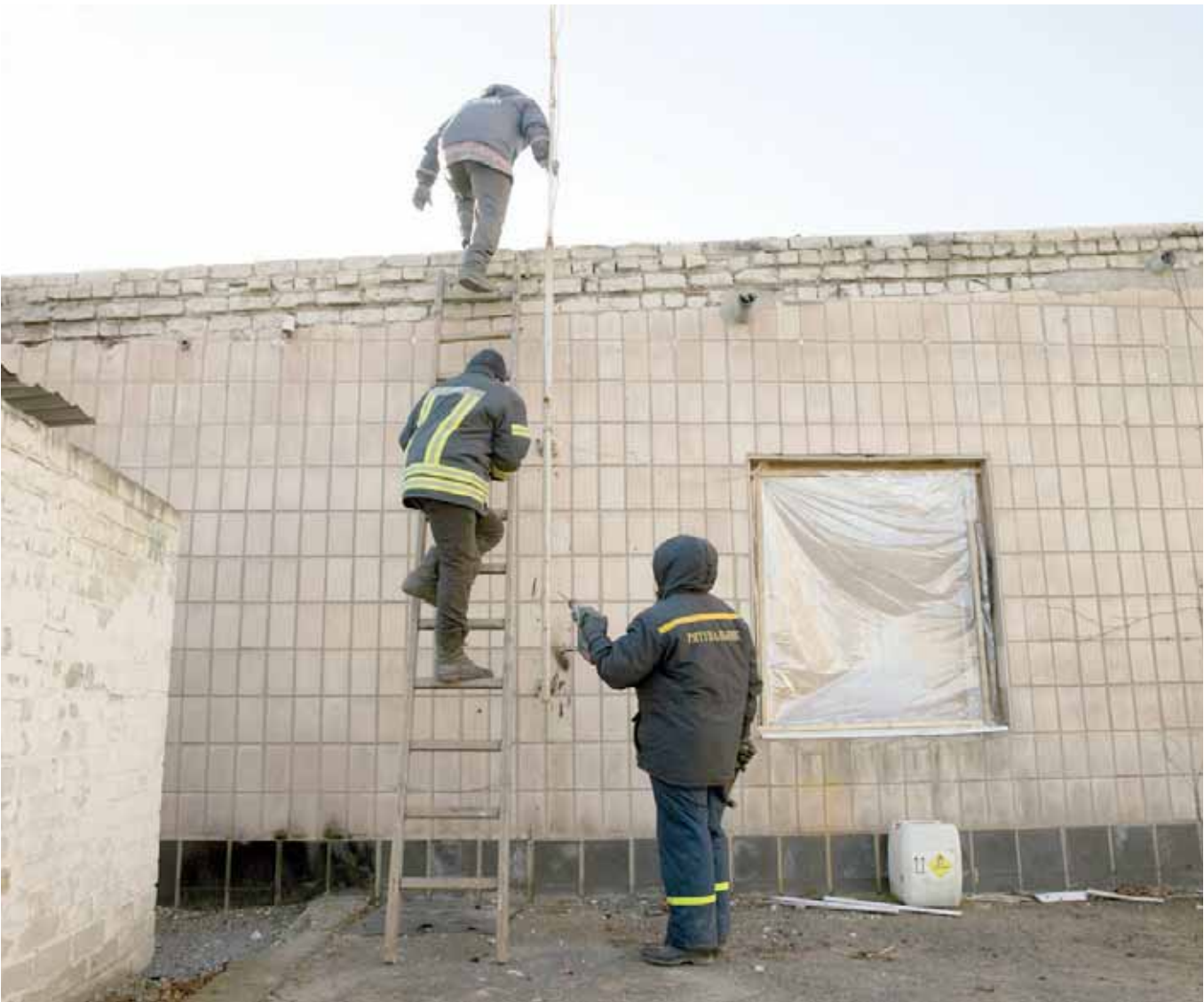
Firefighters from Emergency Service Department Number 21, the single working fire station in Lyman, Ukraine, work to cover up blown-out windows as cold weather grips the country.
