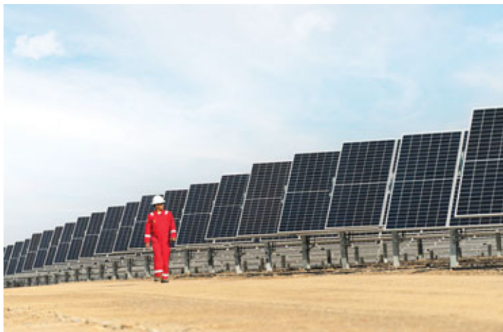
SOLAR MODULES: The plant is located on a 50-hectare site within Sohar Freezone, northern Oman, and consists of over 88,000 solar modules. - Supplied picture
