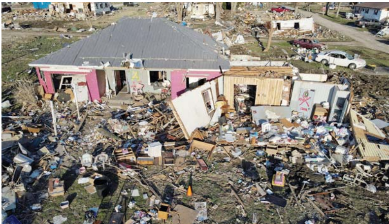
Two severely damaged homes are seen in a neighbourhood in the aftermath of a tornado in Sullivan, Indiana. — Reuters
