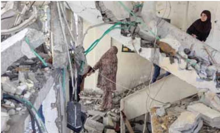
Palestinians inspect the damage in a house after an overnight Israeli strike on Al Daraj neighbourhood in Gaza City on Wednesday. — Reuters
