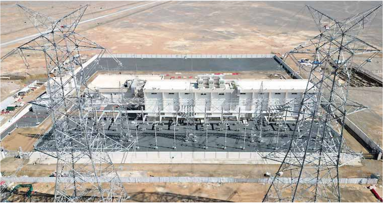
New grid stations are mushrooming all over Oman as part of an expanding national transmission system.
